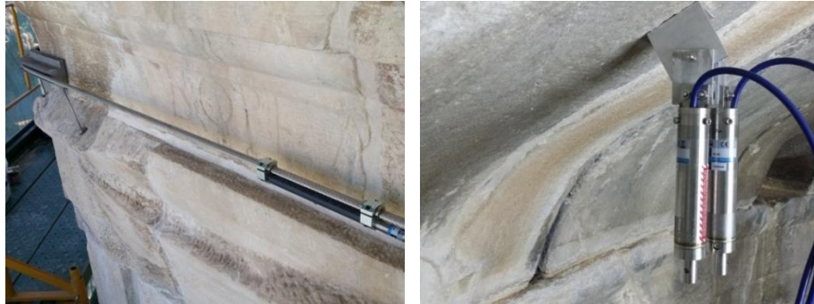
Fig. 3 Sensors currently installed at the Horologion: Extensometer (left) and inclinometer (right)
